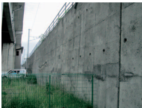
Fig. 2-8 Geosynthetic-reinforced soil retaining wall have a staged constructed full-height rigid facing for Tohoku line (railway), next to Natori River bridge, Sendai City; any damage by this earthquake (photo. by Okamoto, M.)
