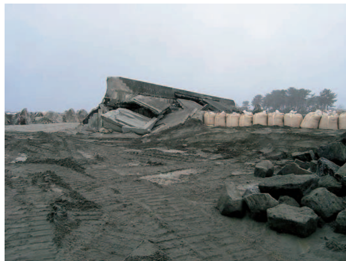
Fig. 13 Destroyed sea wall near Abukuma River mouth
