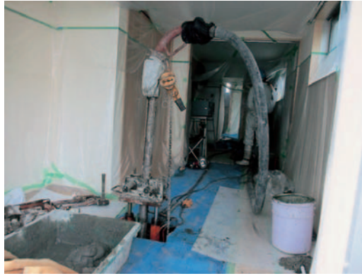
Fig. 3-20 Ground improvement by compaction grouting for restoration of a private house damaged by soil liquefaction, Urayasu City (Yasuda, S.)
