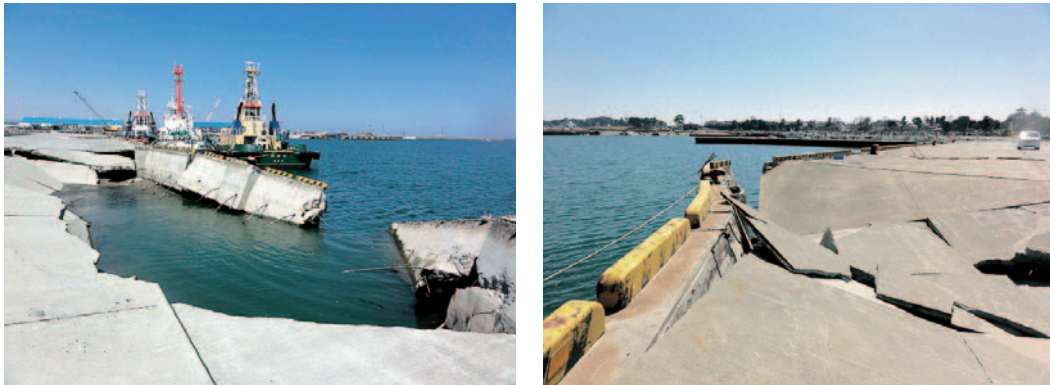
Fig. 3-7 Damage to a sheet pile type quay wall at Soma Port (by the courtesy of PARI)
