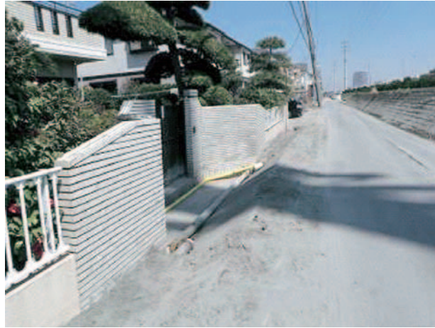
Fig. 3-21 Differential settlements of private house and road, Urayasu City (Ishihara, M.)
