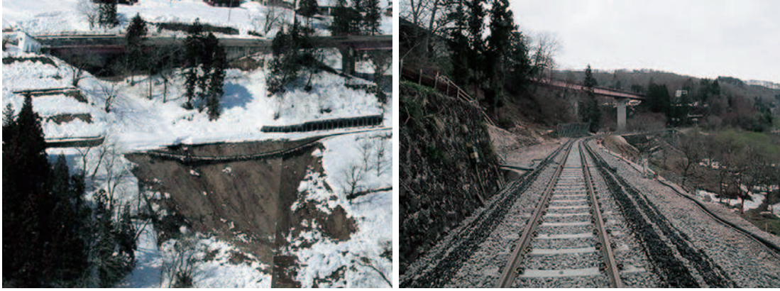
Fig. 3-12 a) Embankment collapsed in the Nagano-Niigata Border Earthquake induced the next day after the 2011 Great earthquake; and b) reconstruction to embankment retained by a GRS-RW having a FHR facing, between Yokokura and Morinomiya, JR East Iiyama Line (by the courtesy of the East Japan Railway Co.)
