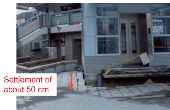
Fig. 3-27 A typical case of ground settlement by soil liquefaction, Urayasu City (Yasuda, S.)
