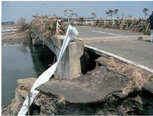
Fig. 11 Erosion of embankment at bridge abutment after tsunami Strike (Iwanuma in Miyagi Prefecture)
