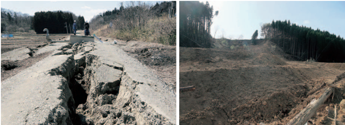
Fig. 15 (left) Damage to a main agricultural pipeline for a length of about 1.4 km due to uplift caused by liquefaction of backfill soil. The largest depth of opening was about 1.6 m (Mohri, H.)
