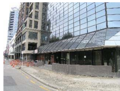
Figure 9 Earthquake damage to a well-designed building (sinking and tilting) caused by unsatisfactory subsoil condition
