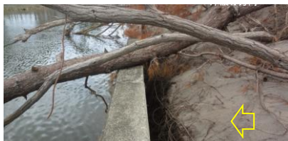
写真-34 貞山堀の矢板護岸の背後の侵食：井土浜③
